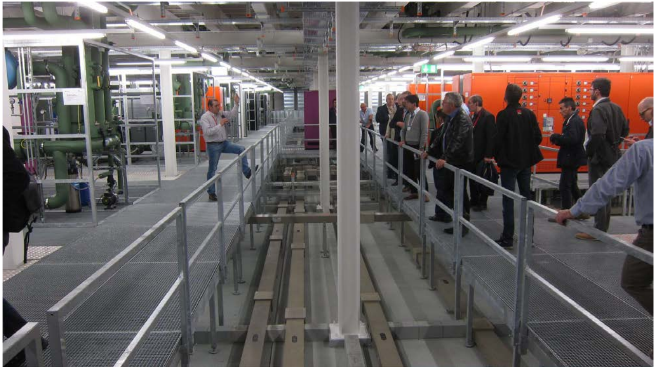
Figure 2: On the installation deck, i.e.: beneath the raised floor
