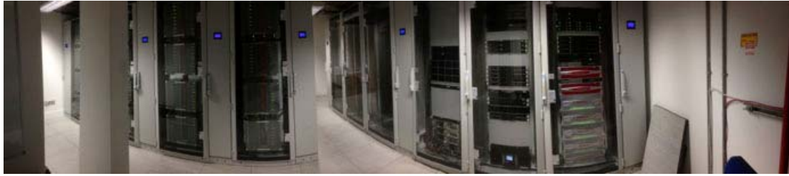
Figure 2 - ICHEC Tier-1 Upgrade system - Fionn
